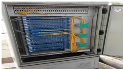
Gambar 5. Optical Distribution Cabinet
